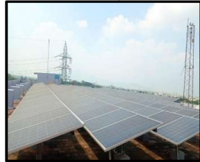
Fig. 5. Aerial view of the solar array traditional installed solar panel
