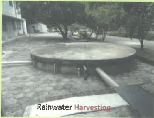
Rainwater collection tank 1 (behind Hostel)
