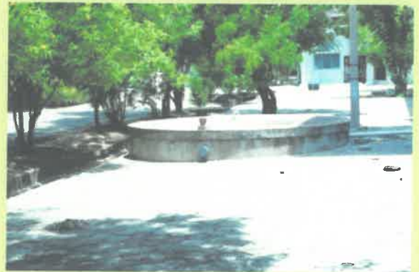
Rainwater collection tank 4 (near Hostel)
