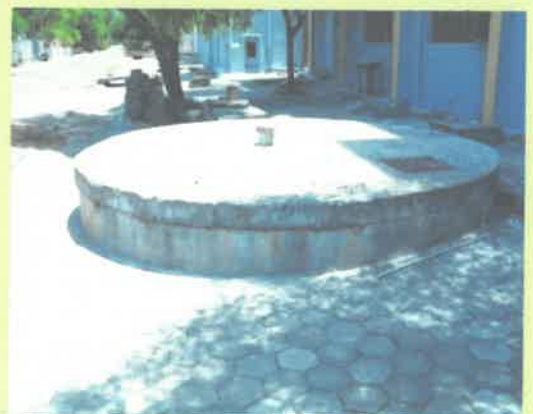
Rainwater collection tank 6 (near School)
