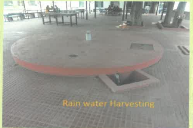
Rainwater collection tank 2 (Food court)
