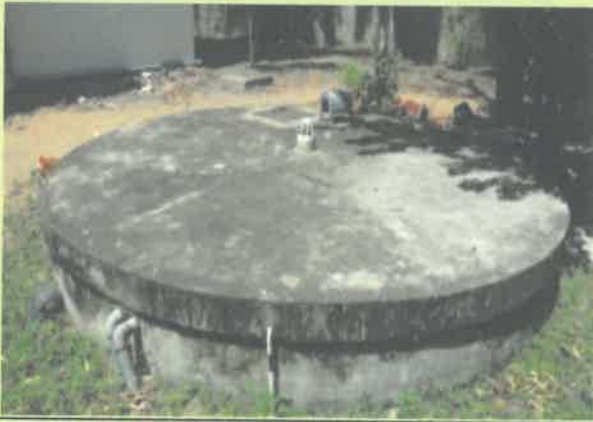
Rainwater collection tank 3 (near Canteen)
