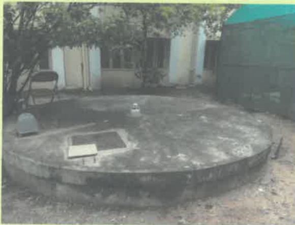
Rainwater collection tank 5 (near Green house)
