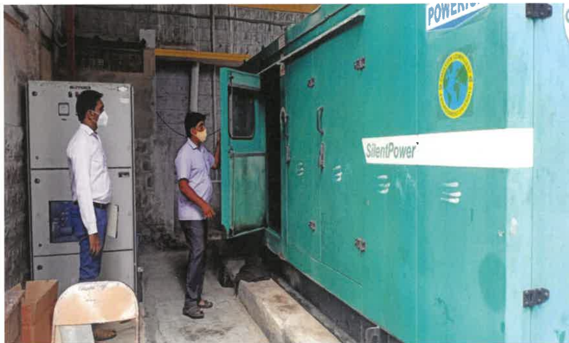
Generator Installed at Campus -I
