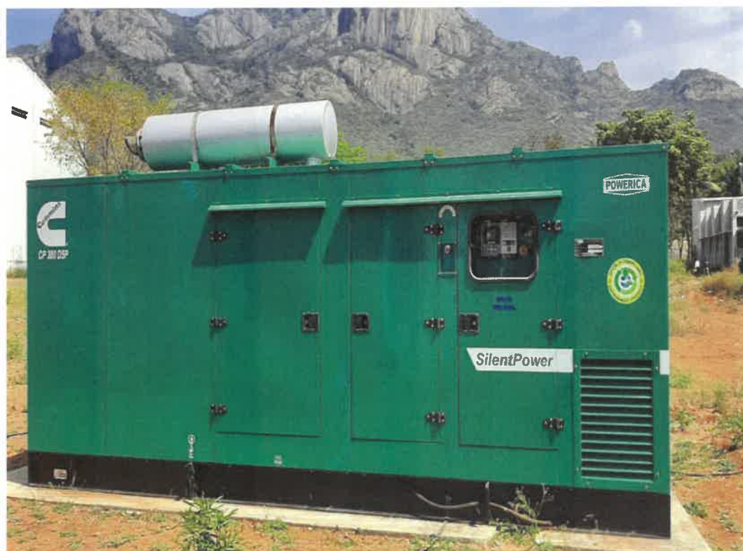
Generator Back up at Campus II
