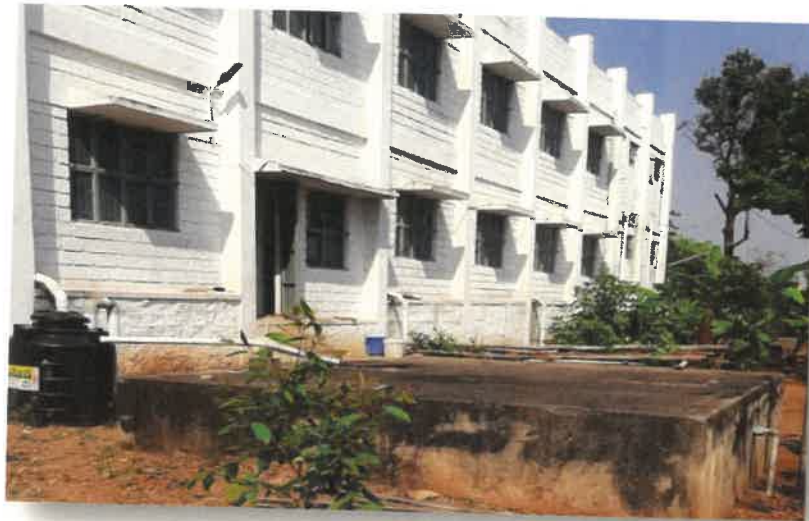
Rain Water collection tank (Campus II)
