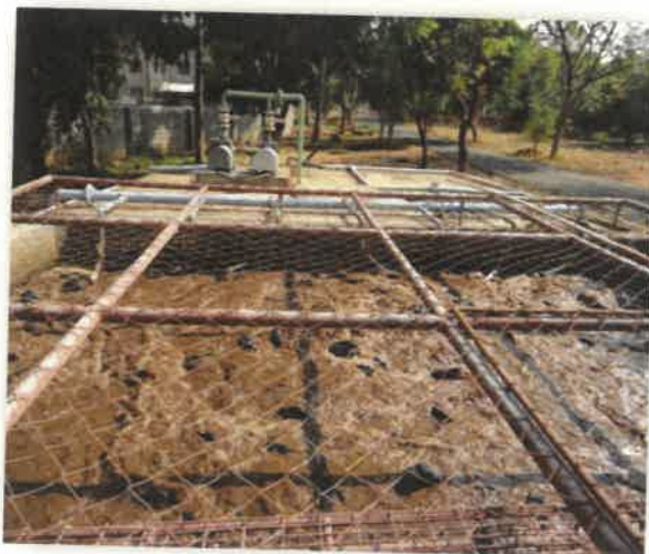
Sewage treatment plant (STP)
