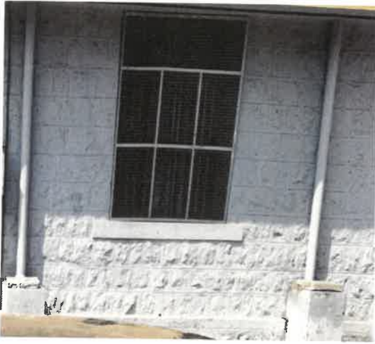
Rain water collection (Campus I)
