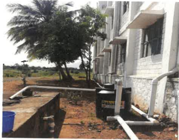
Rain water collection (Hostel-Campus II)
